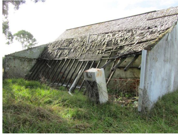
VIEW OF THE COLLAPSED REAR SKILLION ROOF AND REMNANT TIMBER SHINGLED ROOF
