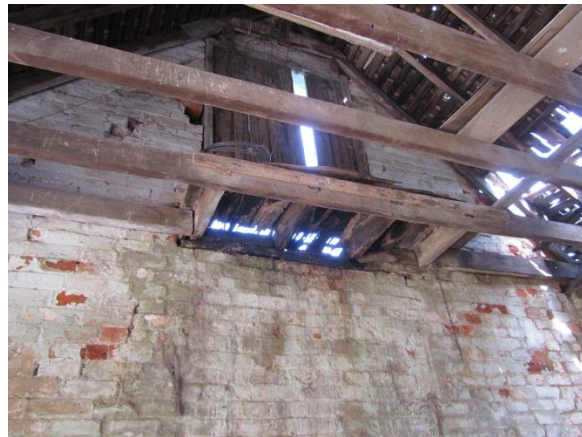
REMNANT TIMBER ROOF STRUCTURE AND REMNANT TIMBER SHINGLES
